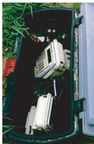
Figure 6.15 Sigma bubbler flowmeter at USGS test site.
