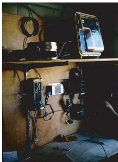
Figure 5.27 Telemetry equipment at USGS monitoring site in Madison, WI.
