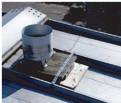
Figure 6.53 Rain temperature monitoring by WI DNR in Madison, WI.
