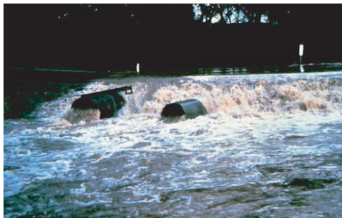
Figure 4.5 High flows in Coyote Creek overtopping road culvert.
