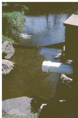
Figure 4.19 Stilling well at Bellevue flow monitoring station.
