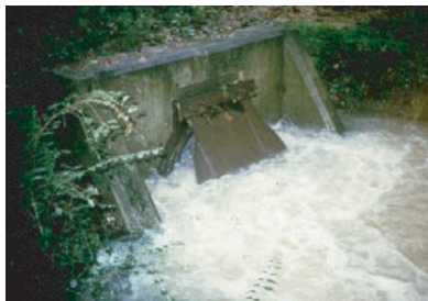
Figure 4.44 Five-Mile Creek SSO discharge during large flow.
