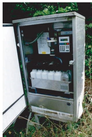
Figure 5.29 Automatic sampler connected to continuous probes and telemetry at Dortmund, Germany.
