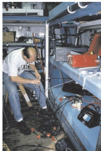
Figure 3.4 Installation of side-stream fish bioassay test facilities at Lincoln Creek, Milwaukee, WI.
