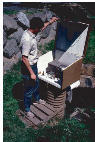
Figure 4.20 Level recorder at Bellevue flow monitoring station.
