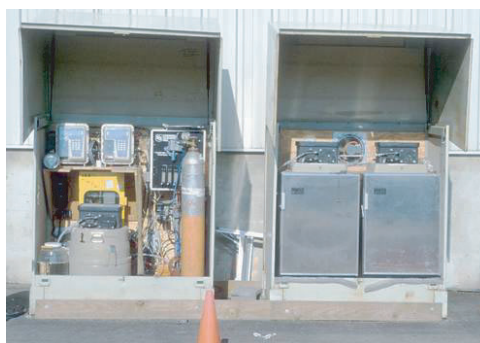
Figure 5.26 .Multiple flow monitor and sampler setup for simultaneously monitoring influent and effluent over wide range of flow conditions at a small treatment device in Madison, WI.
