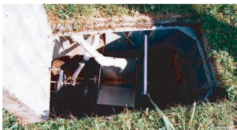
Figure 6.35 Tipping bucket flow measurement device for measuring groundwater flows at UW test plot.
