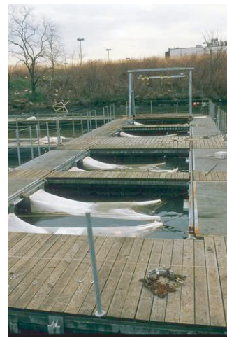
Figure 3.26 New York City's use of end-of-pipe TrashTrap systems.
