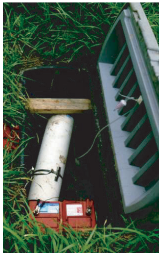
Figure 6.17 Acoustic flowmeter at USGS test site.
